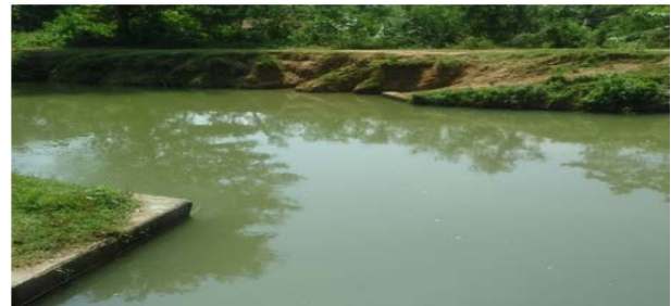
Figure 1. extensively eroded downstream canal banks just after a hydraulic structure in one of the Walawe right bank canal.
