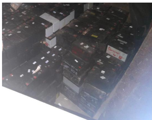
Figure 2.4: Disposal of UPS batteries
